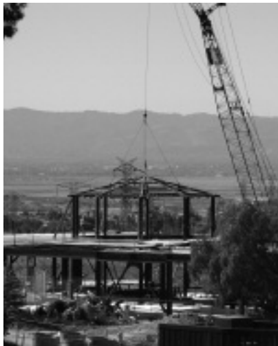
The rotunda for the new Student Support Services Building is put in place in March 2008. Photo courtesy of College Advancement.
