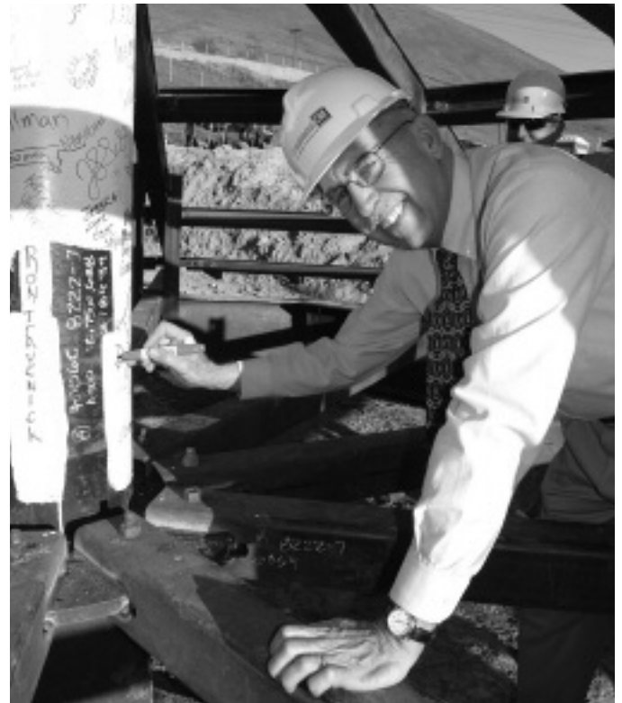
Past Ohlone President Doug Treadway signs the rotunda beam for the new Student Support Services Building. Photo courtesy of College Advancement.
