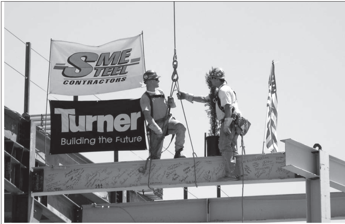
Ironworkers secure the final metal beam in the new Newark campus building in last week's "topping off" ceremony.
