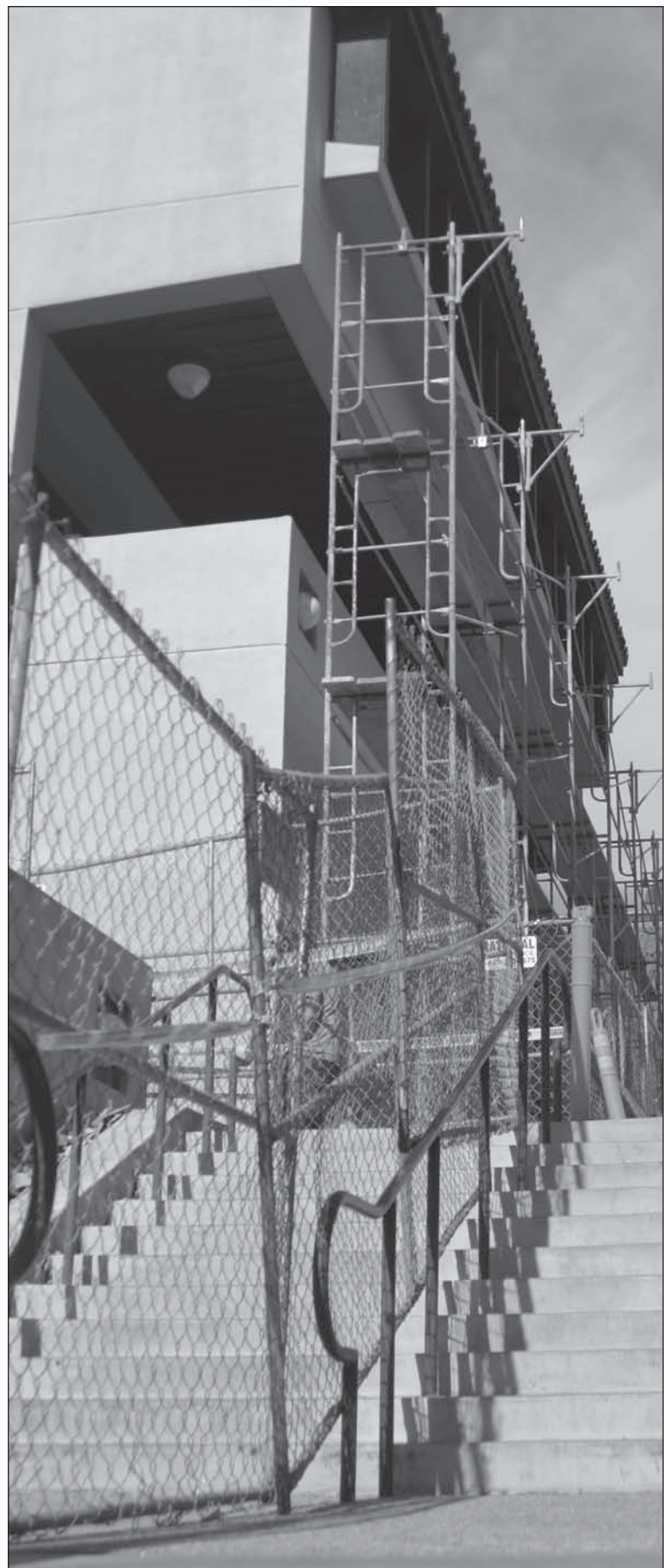
Photo by Christa Meier Scaffolds, walkways, shadows form geometric patterns on Ohlone buildings during construction period.
